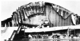
The collapsed roof of the Congress Hall, 1980.
